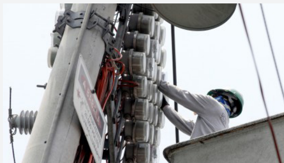
ROUTINE INSPECTION. Workers of power distribution utility Manila Electric Co. conduct a routine inspection of overhead electric power meters along Road 10 in Tondo, Manila on April 23, 2026. Senate President Win Gatchalian on Monday (July 13) asked the Energy Regulatory Commission to consider spreading out Meralco's July electricity rate increase to spare households and small businesses from a sudden spike in their monthly bills. (PNA photo by Yancy Lim)
